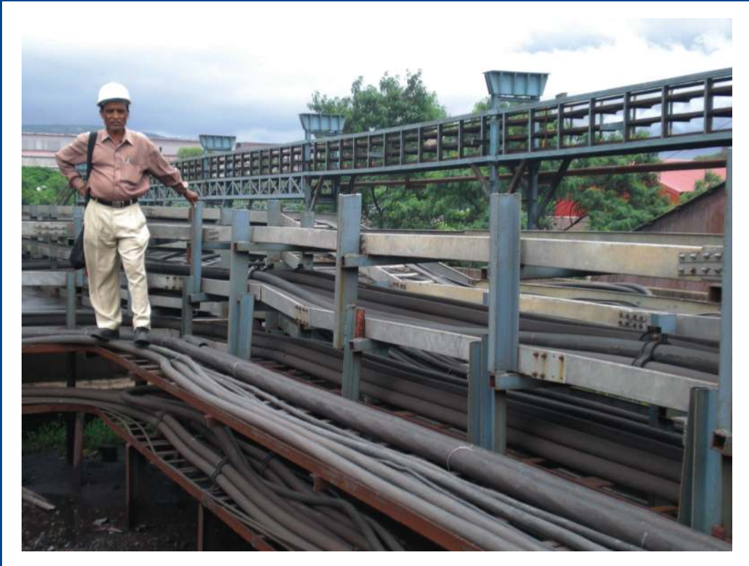
Fabrication and erection of cable Trays and laying of cables at JSPL Raigarh Contract No.478001842
