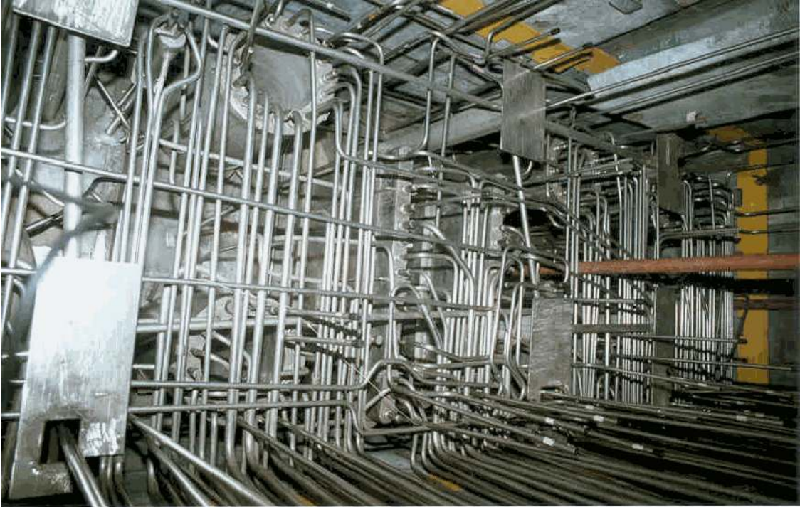
Quality Control works for ABB at Mussafah in Abu Dhabi, UAE at Contract No.A65.6001/OH1/rs
