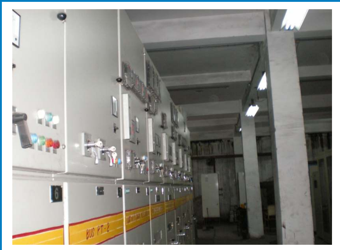
Electrical Jobs for New 25MW Chinese TG at JSPL Raigarh Contract No.4778001677
